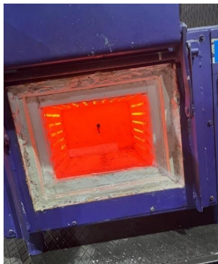
Figure 2.8: Electric resistance heat treatment furnace
